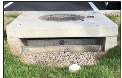
REAR VIEW OF OUTLET SCREEN
